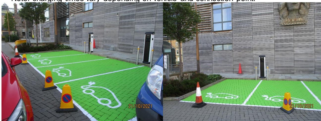
Images of free standing dual EV charging units, with marked parking bays, installed at Helensburgh and Lomond Civic Centre
